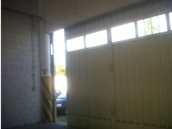
PORTON INGRESO VEHICULOS
